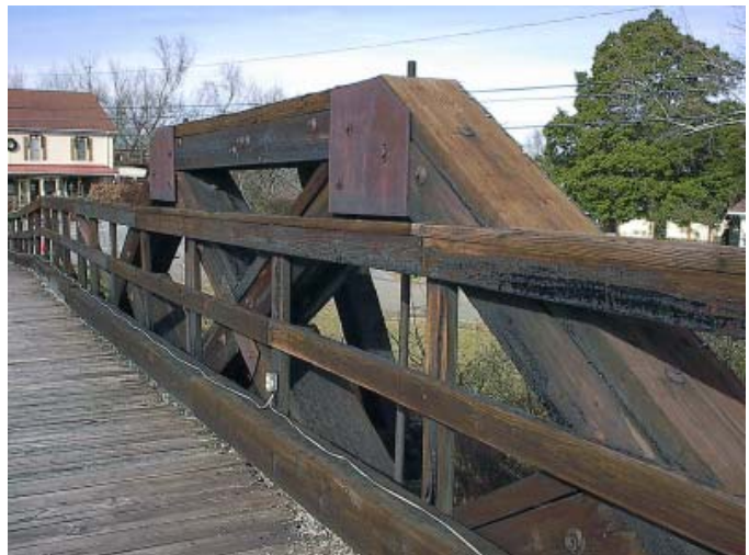
Γέφυρα Chambers Street
