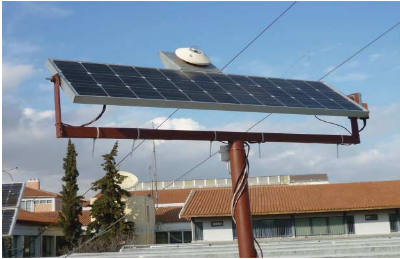
Figure 1. The photovoltaic panel.
