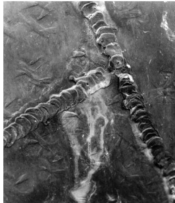
Fig. 12: Example of galvanic corrosion on welds.
