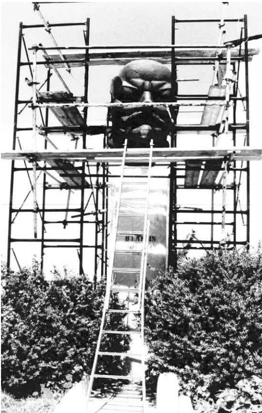
Fig. 13. The monument with the scaffolding placed for the implementation of the conservation work.
