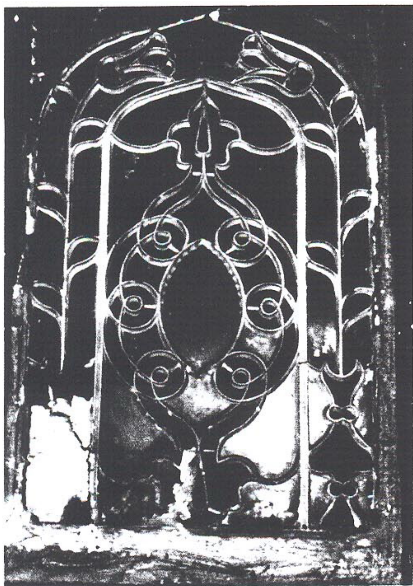
Fig. 2. Detail of weathered glass window.
